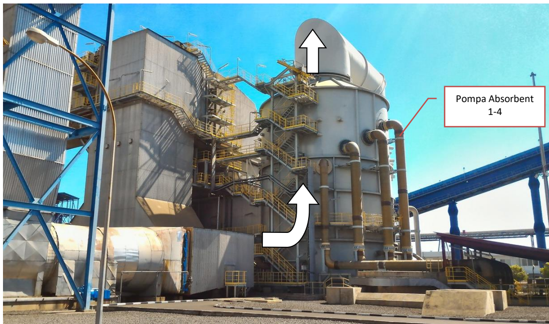
Gambar 1. Sistem FGD di PLTU paition Unit 5 & 6 PT. Jawa Power
